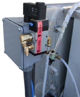
Figure 6. Tank Dump Solenoid on Skid
